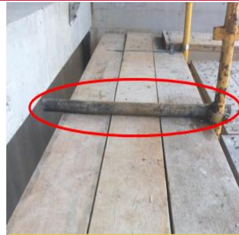
Support Tube, which had been removed by scaffolder
