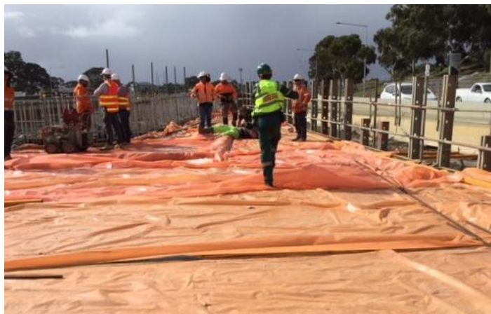
Plastic sheeting covering unidentified hazards underneath
