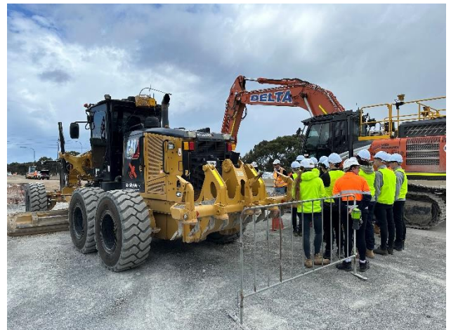
Aldinga High School students learning about plant and equipment used on the Majors Road Interchange Project.
