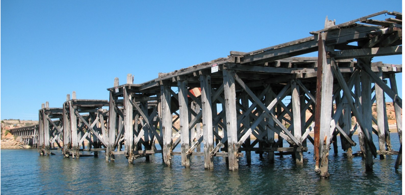
Image: The old Wardang Island boat landing facility, demolished in 2007 due to its deteriorating condition.
