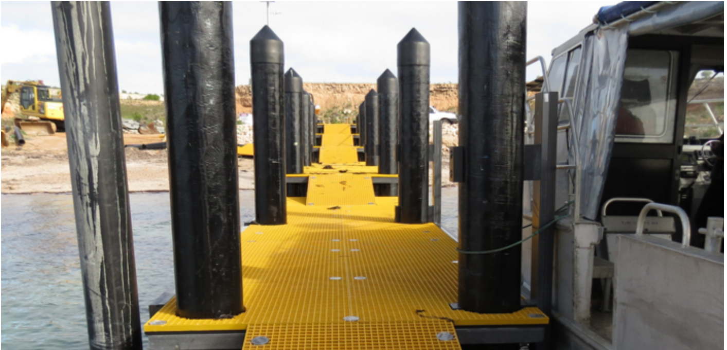
Image: A new type of composite fibre reinforced plastic grating decking was used for the jetty. The decking has an anti-slip coated surface, is yellow in colour to ensure its visibility and is designed to be low maintenance, durable and last a long life span.
