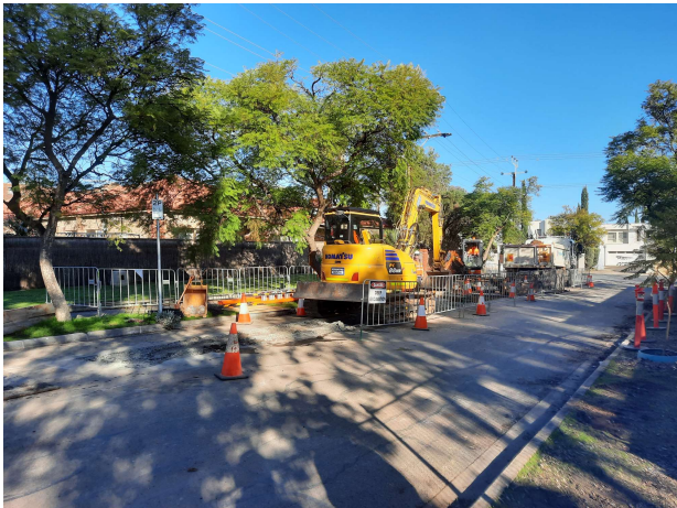
Image: Trenching Works as part of the Glen Osmond Road and Fullarton Road Intersection Upgrade
